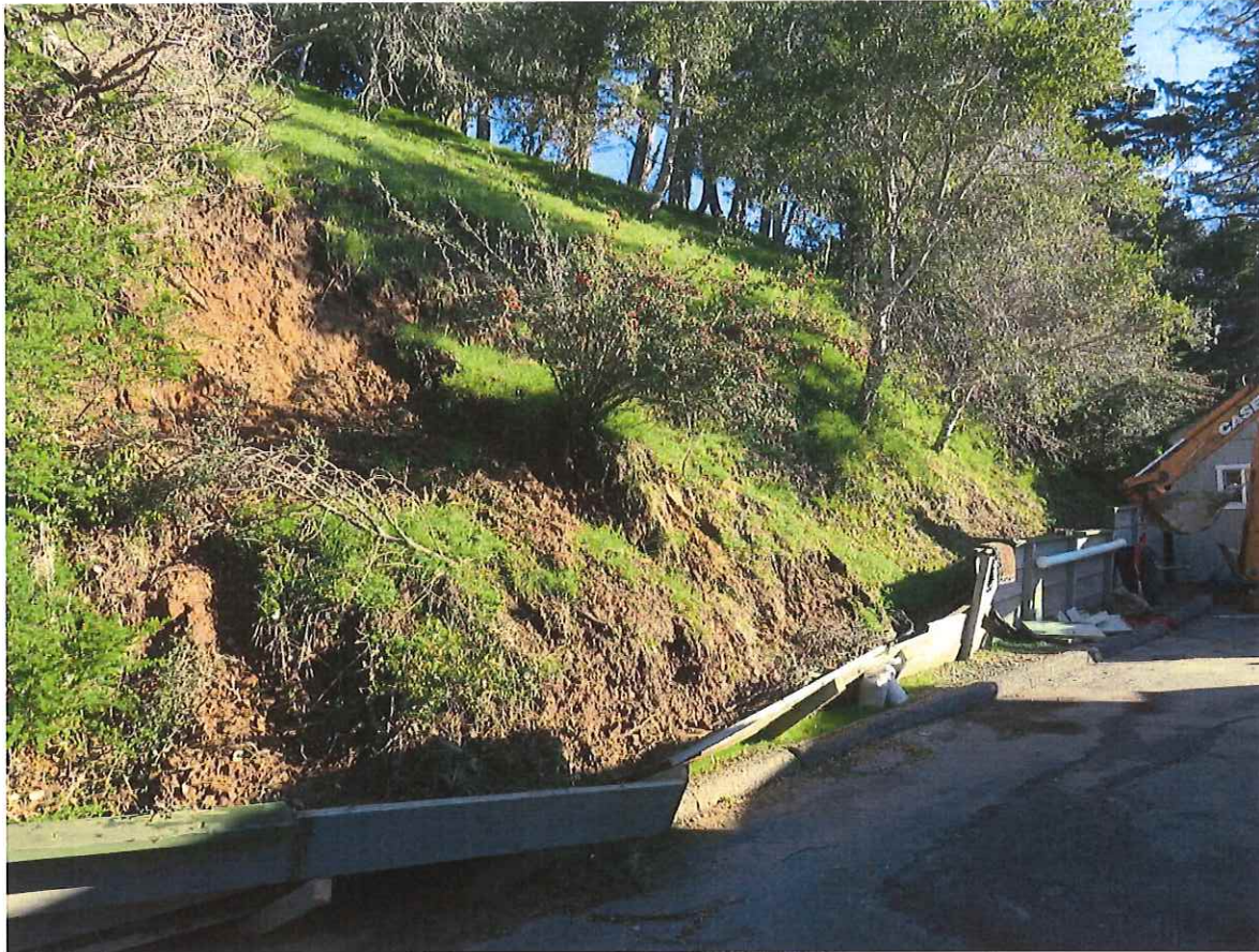
Figure 4: View northeast of failure of cut slope. Note proximity of building in back to cut slope and failure of wood wall. Trench T-1 was excavated near the building, Trench T-2 was excavated in the slide, and Trench T-3 was excavated just left of the sight of the picture.
