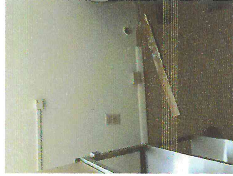
Building: Suite A 2511, Room: 31 Hall, Element Id: ER1-01
