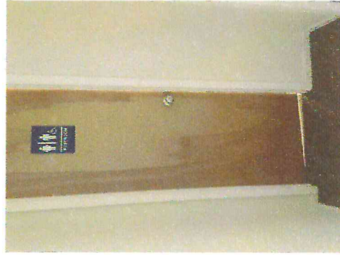
Building: Suite A 2511, Room: 27 Toilet Room, Element Id: DRSW1-01
