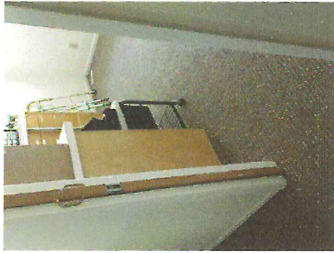
Building: Suite A 2511, Room: 29 Storage, Building: Suite A 2511, Room: 30 Exam, Element Id: DRNO 1-01
