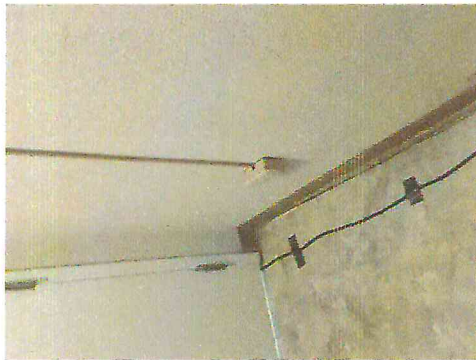
Building: Suite B and C Clinic 2515B, Room: 7 Rear Entry, Element Id: ER1-01
