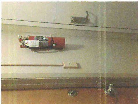
Building: Suite B and C Clinic 2515B, Room: 7 Rear Entry, Element Id: FE1-01
