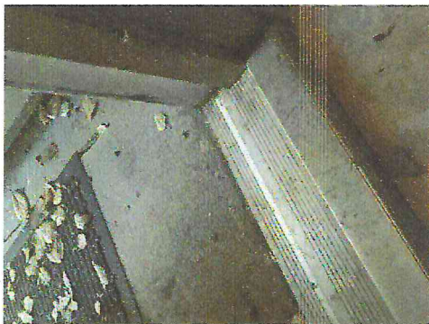
Building: Suite B and C Clinic 2515B, Room: 7 Rear Entry, Element Id: DRSW1-
